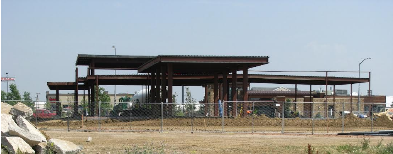
First Interstate Bank Under Construction at Intersection of Lakeway Road and South Douglas Highway
